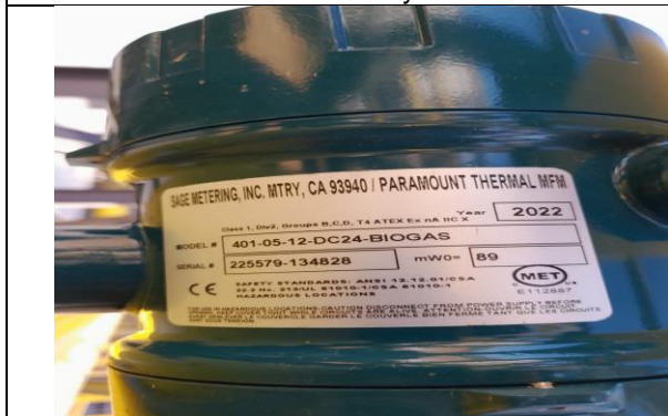
Gas engine flowmeter
