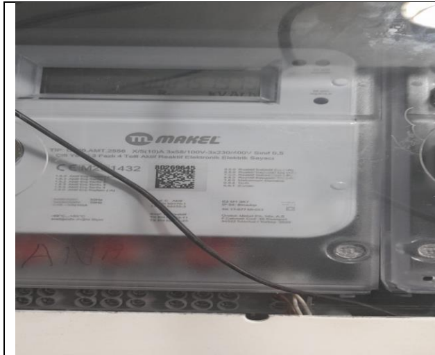
Main electricity meter
