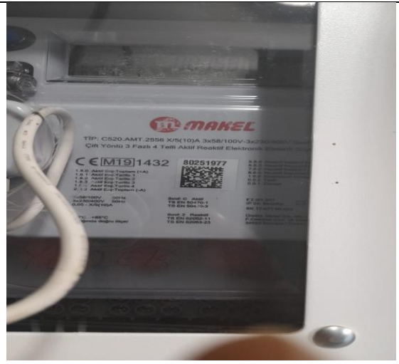
Spare electricity meter
