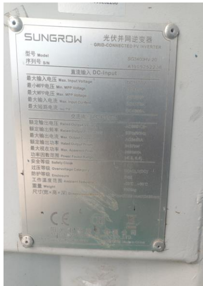
Inverter Name Plate Verification
