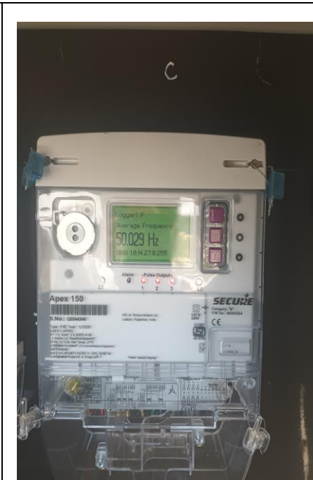
Monitoring Equipment (Check meter installed at site)
