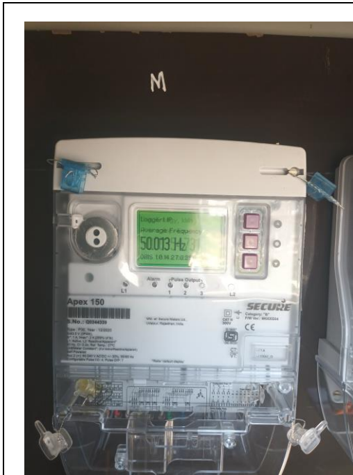
Monitoring Equipment (Bidirectional Energy Meter) installed at site)-Main Meter
